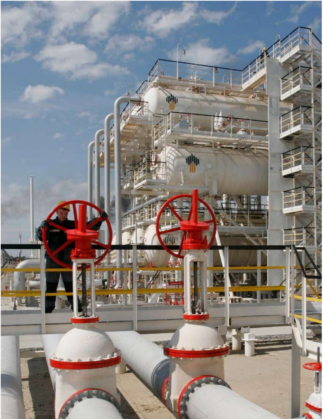
Separation unit at Central Treatment Facility – 8, Yuganskneftegaz
